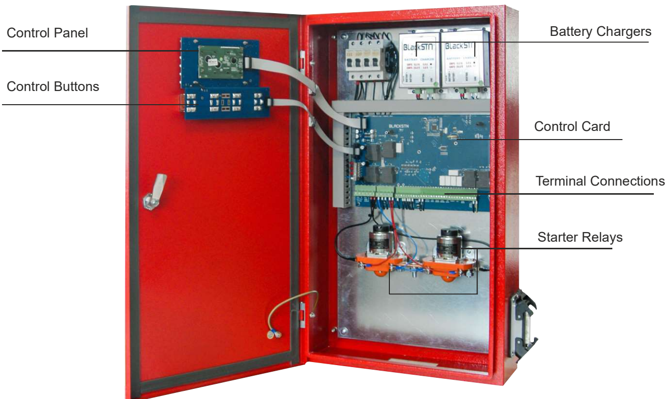
Figure 1: NFPA 20 Diesel Fire Panel Inner View
