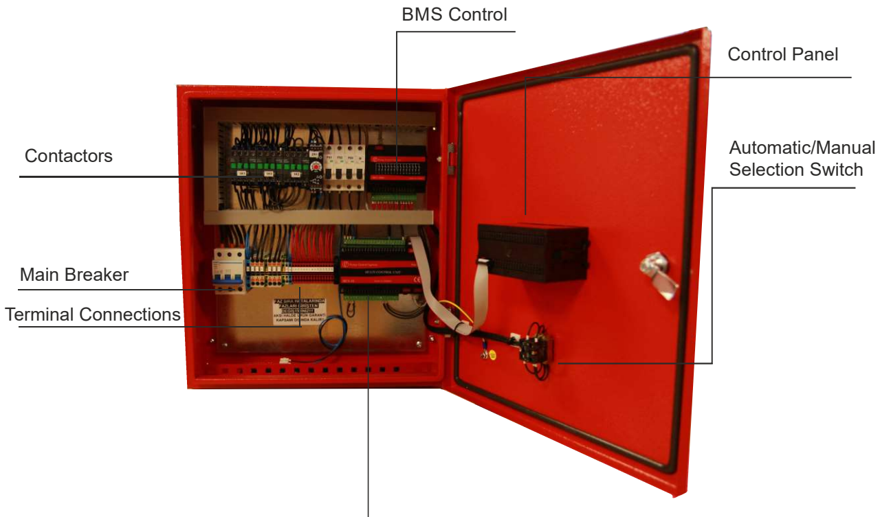
Figure 1: NFPA 20 Electrical Fire Panel Inner View
